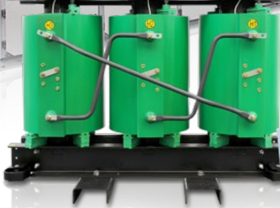
Dry Phase Shifting Transformer
